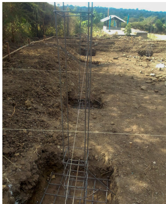
Column setting of the treatment plant at Oloolaiser Water and Sanitation Company in Kajiado County.
