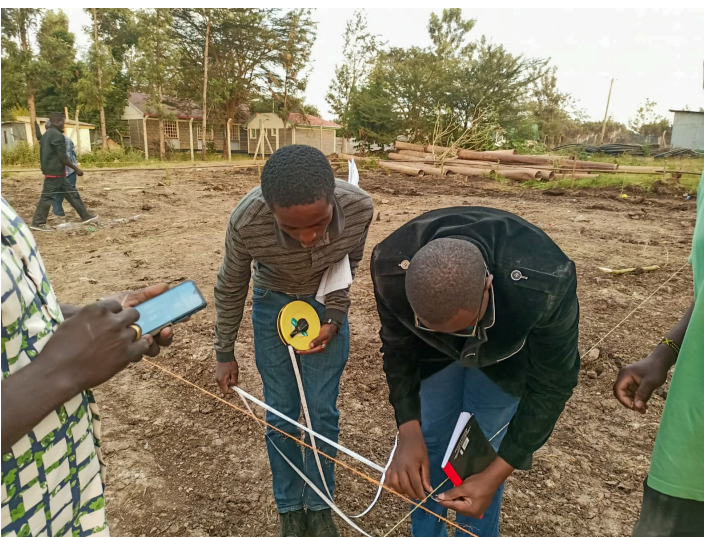
Mr. Seth Muthusi, KEWI Quality Assurance Officer checks measurements during the construction of the GTS.
