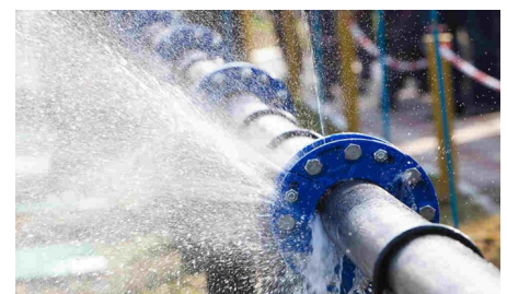
A leaked pipe.
