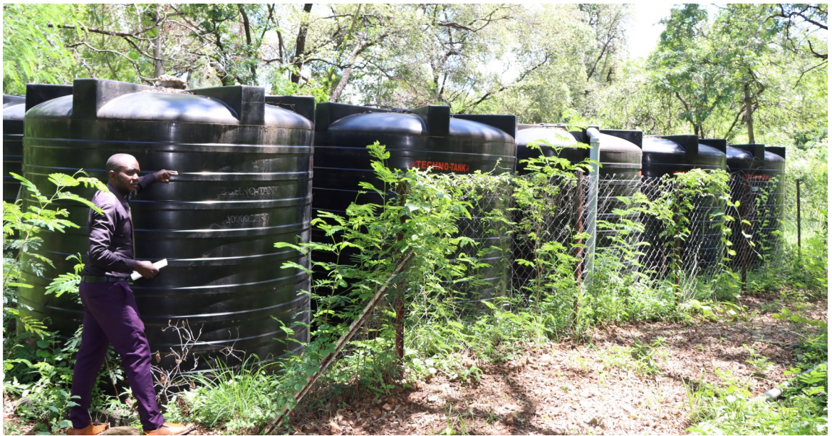
Water storage tanks in Chiakariga Campus. The Campus has adopted water harvesting techniques. The Campus is located in one of the Semi Arid areas in Kenya, in Tharaka Nithi County.
