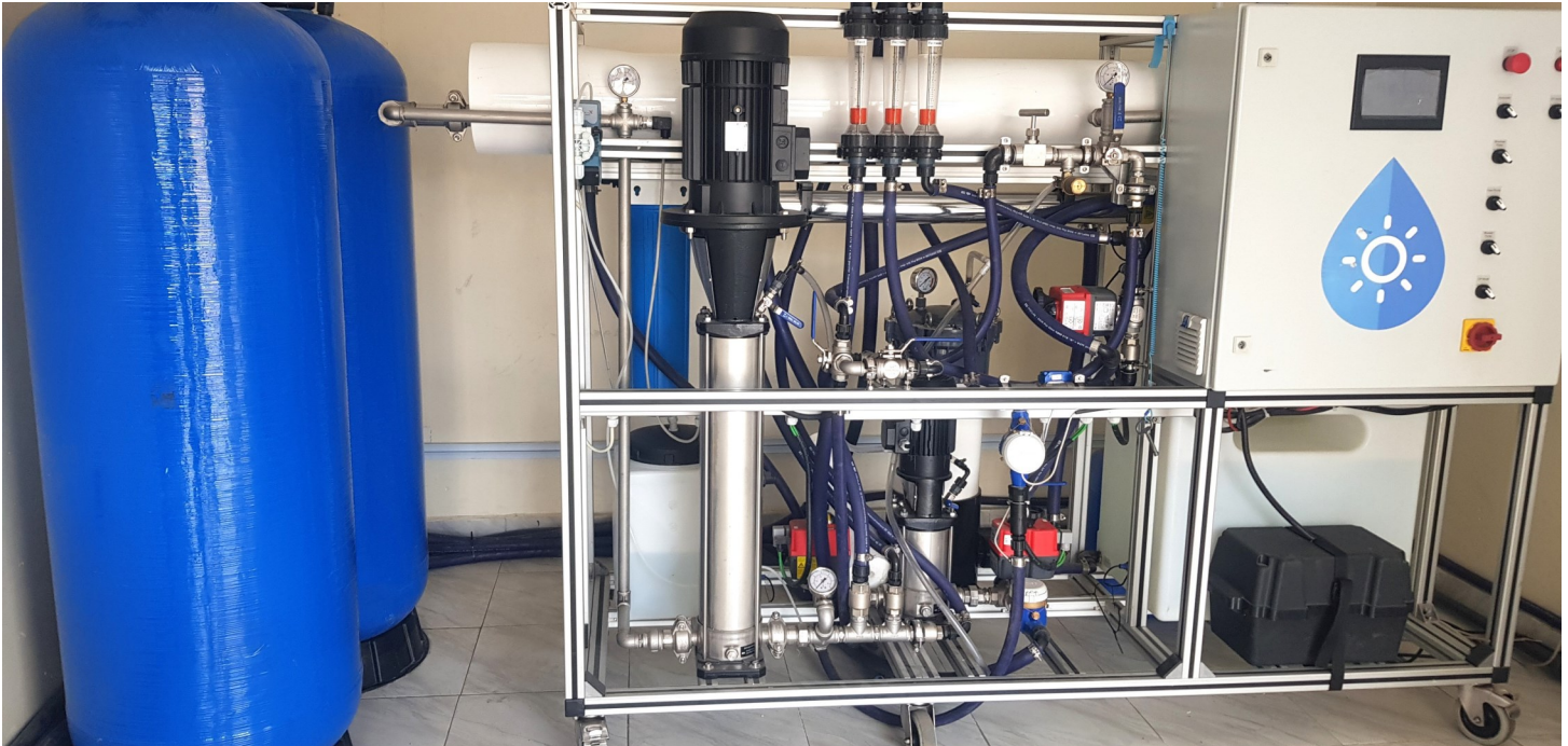
A water desalination plant coming up at KEWI headquarters, Nairobi. This is a joint project between KEWI and Water Kiosk Africa.
