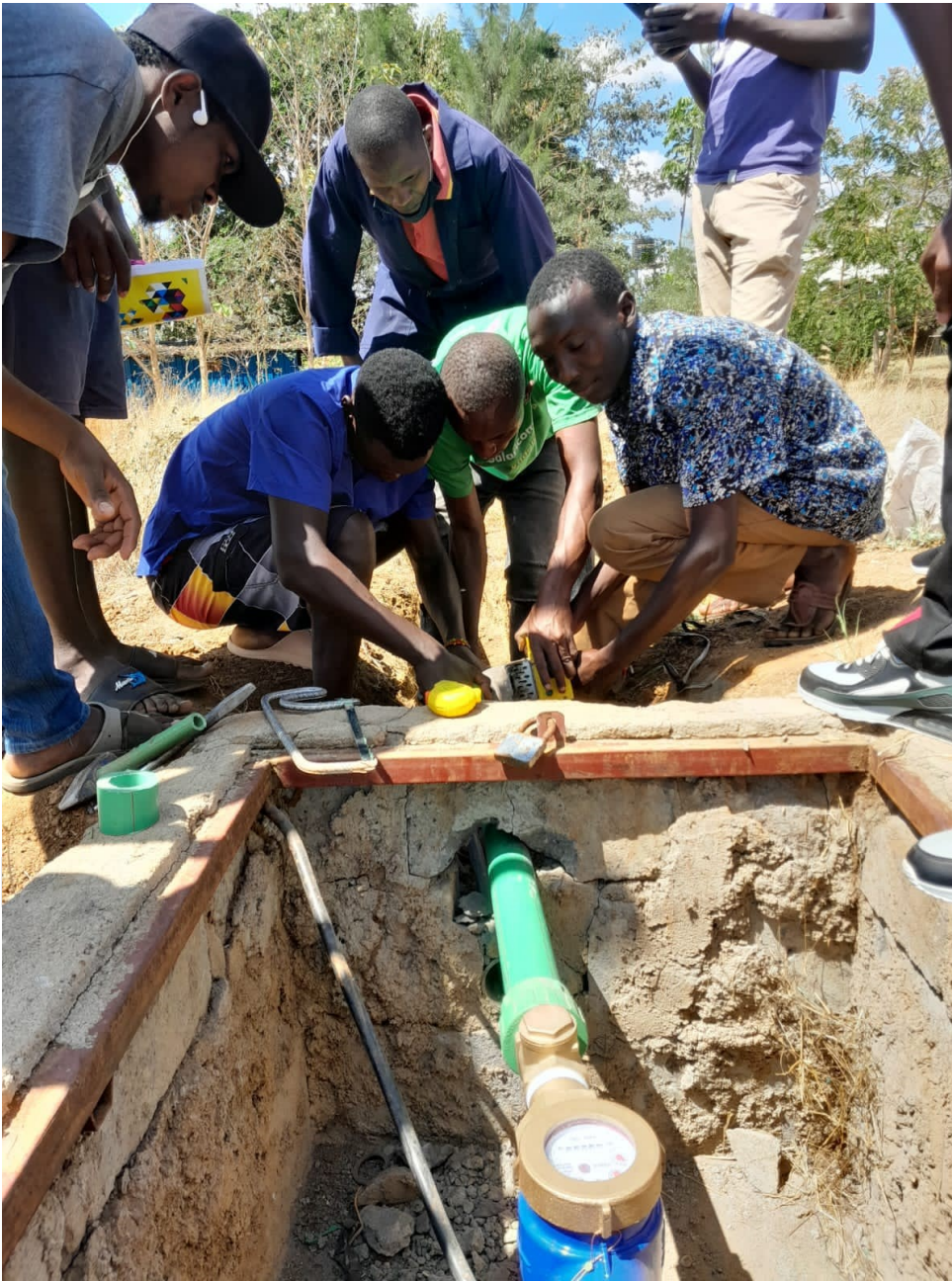
Students from Kitui Campus in a practical pipe-laying exercise at the campus.
