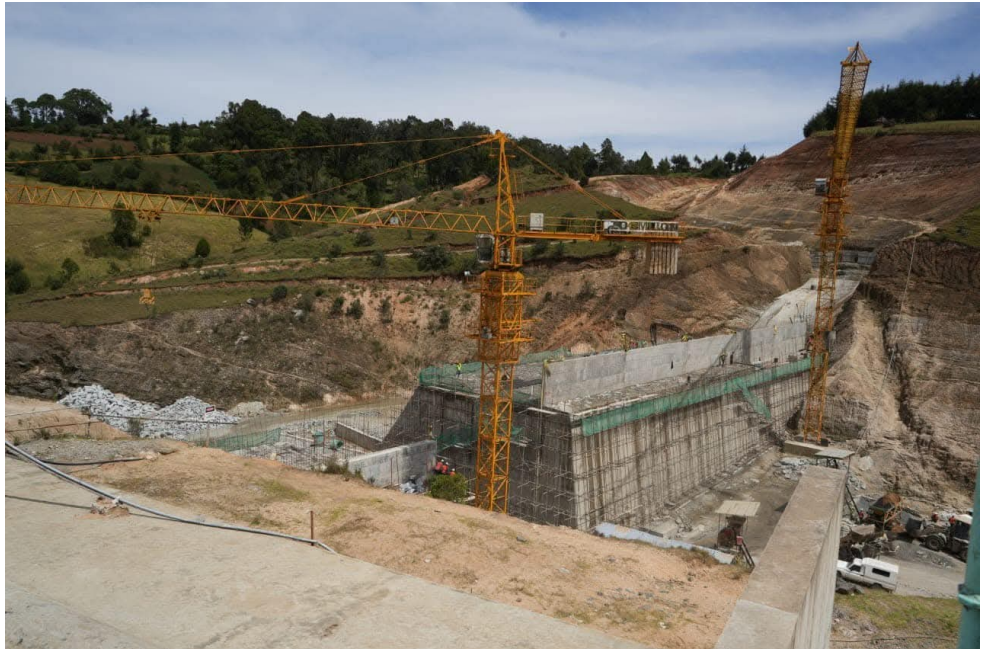
Muruny (Siyoi) Dam project under construction in West Pokot County. Realization of mega projects in the ministry requires joint financing efforts between the public and private sector and thus the need for Public-Private-Partnership (PPP) financing model. (Photo: Ministry of Water, Sanitation and Irrigation)
