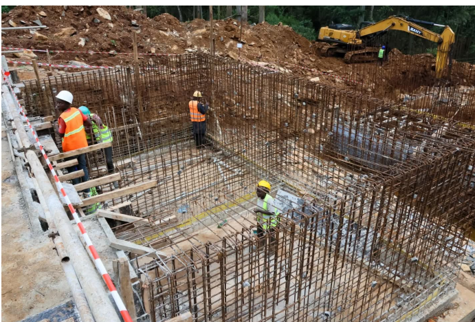
Ongoing construction of Kabianga Water Supply Project in Belgut Constituency, Kericho County (Photo: Ministry of Water, Sanitation and Irrigation)
