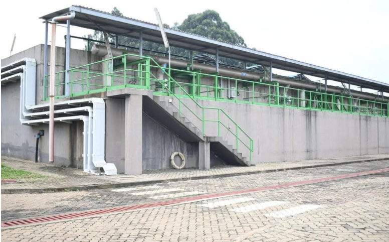
Section of the Northern Collector Tunnel Project which is part of the Nairobi Water Master Plan, a component of the Fourth Nairobi Bulk Water Supply System. (Photo: Ministry of Water, Sanitation and Irrigation)
