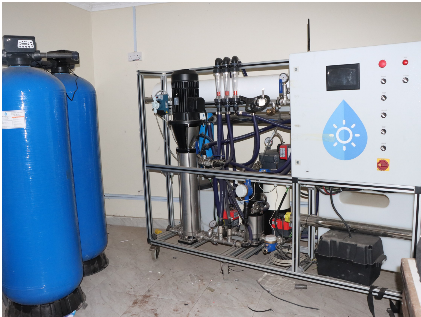
A solar water desalination plant at KEWI.
