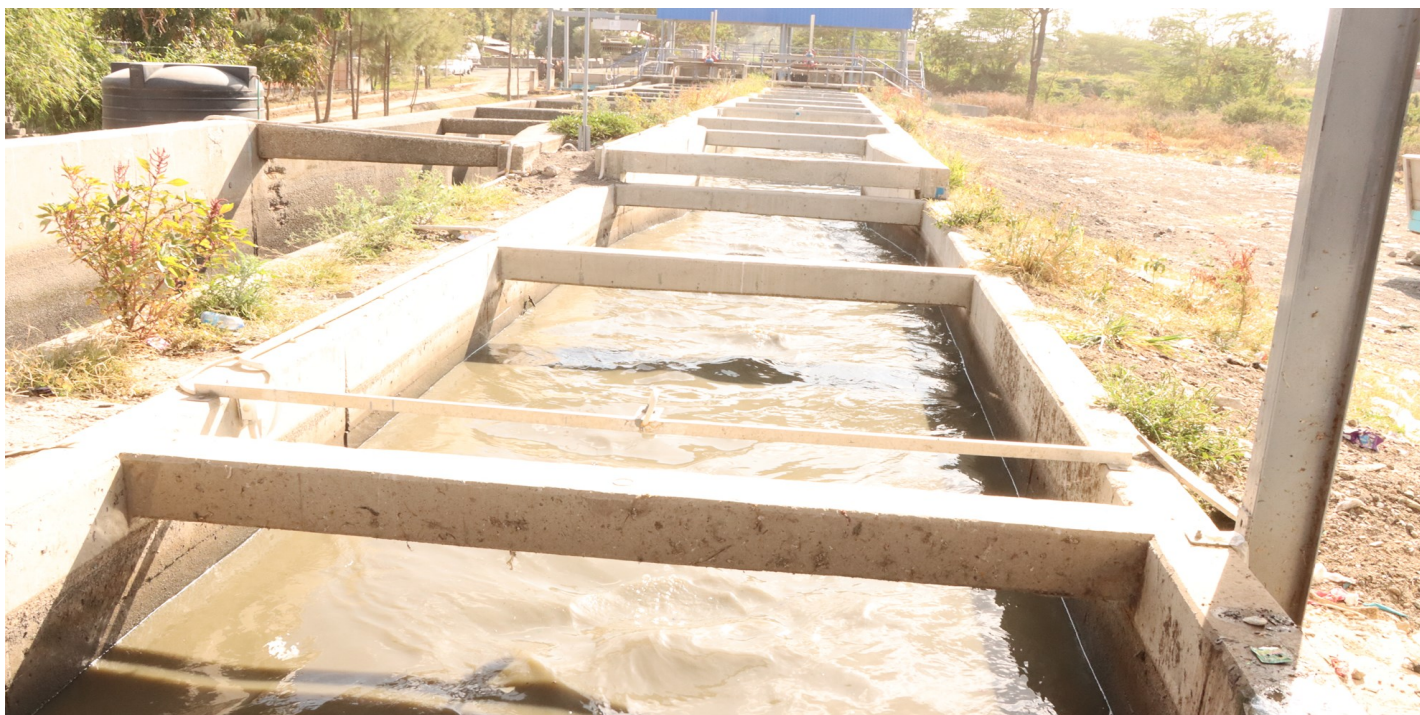
A Sewage Tunnel at the Dandora Estate Waste Water Treatment Plant.
