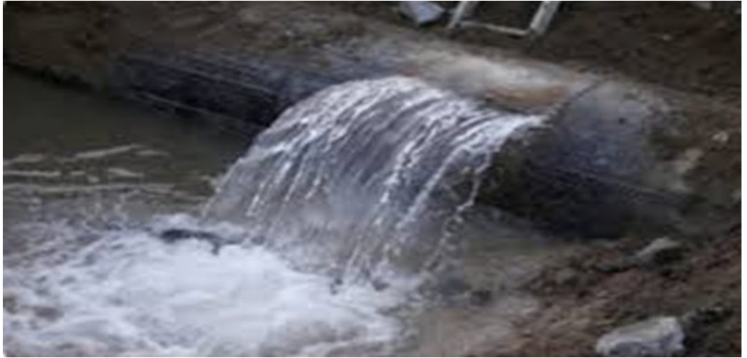
A leaking water pipe. 32 billion cubic meters of water are lost through pipe bursts .
