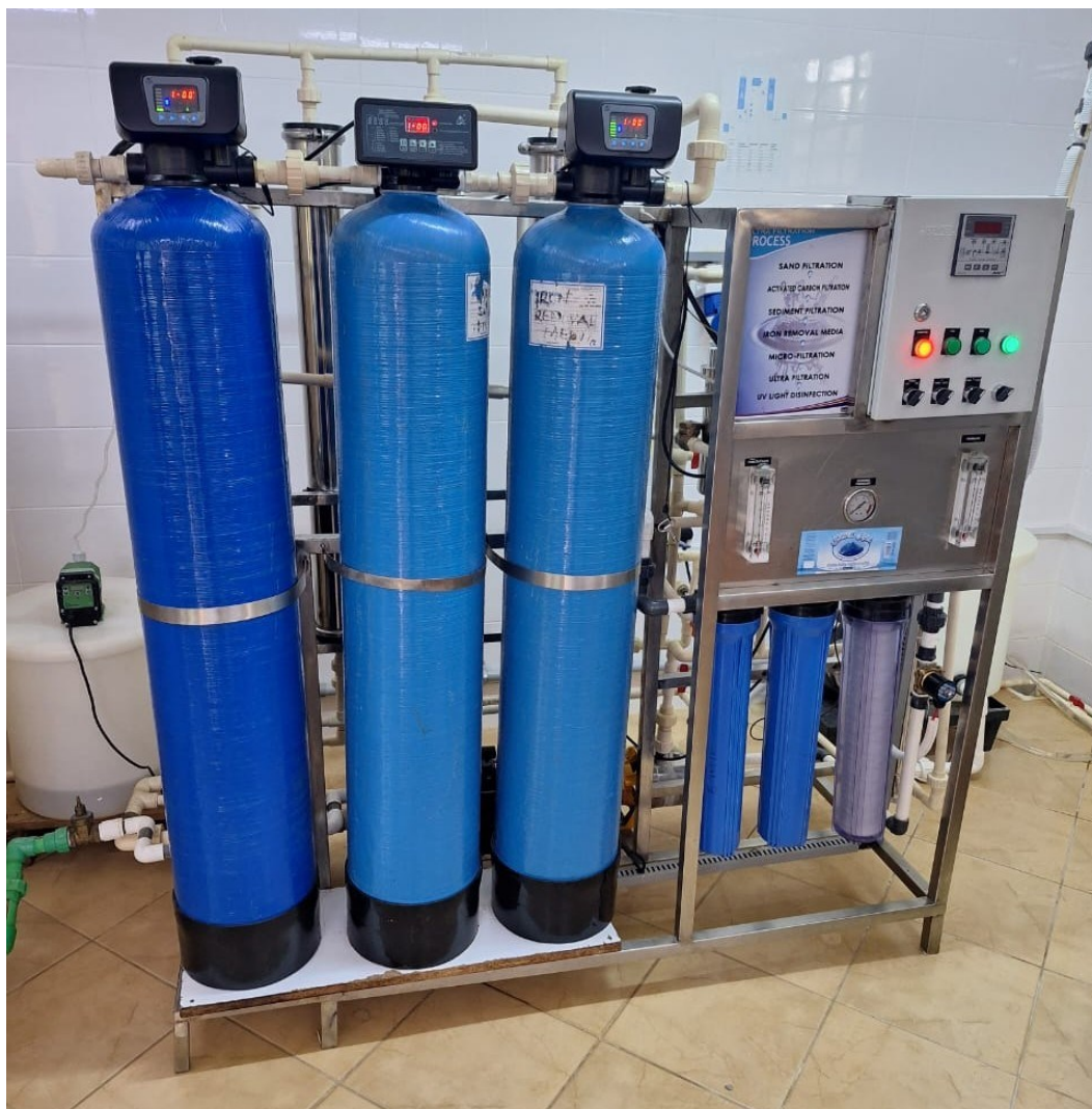
A water purification plant at Horizon Aqua Water Bottling Company, Vihiga County.
