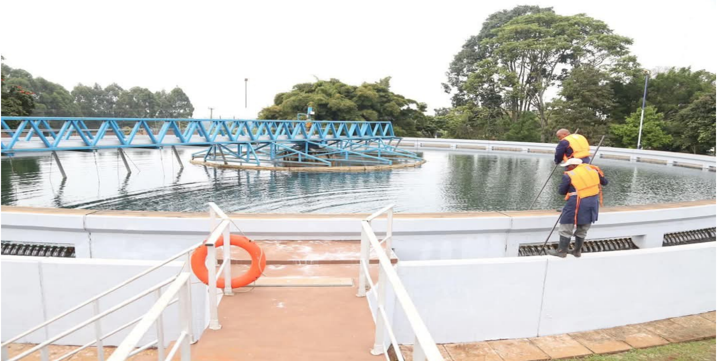
Workers during one of their maintenance routine at Ngethu Water Treatment Plant in Kiambu.
