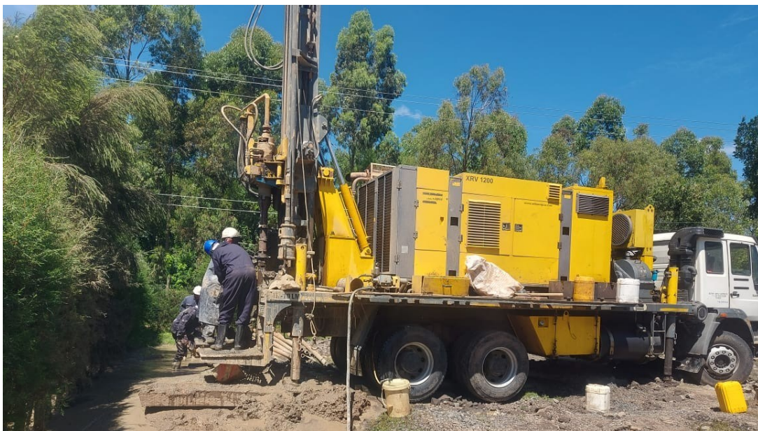
KEWI borehole drilling rig in the field. KEWI is directly involved in borehole drilling, ensuring that the work is done according to professional standards
