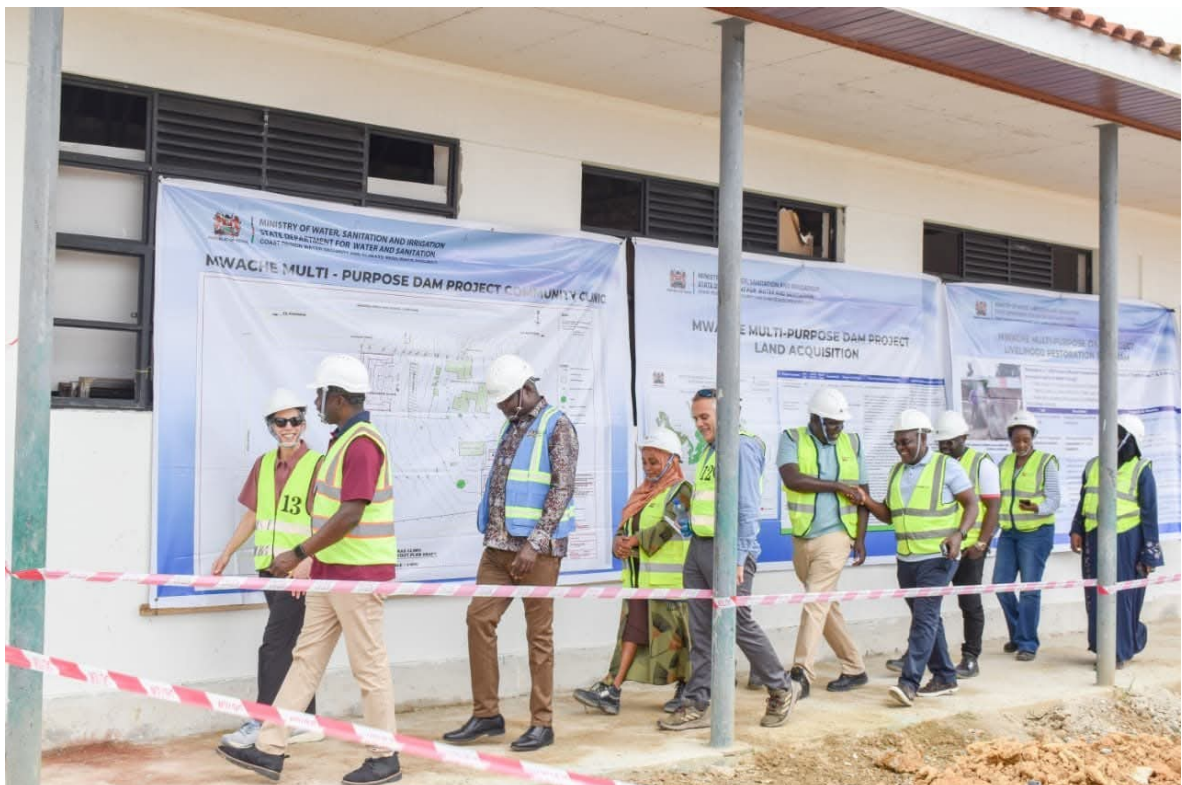
PS Korir, CBS with World Bank Task Force team and the Project Management Unit, for a special visit to the Mwache Multipurpose Dam Project site in Fulugani Village, Kwale County.
