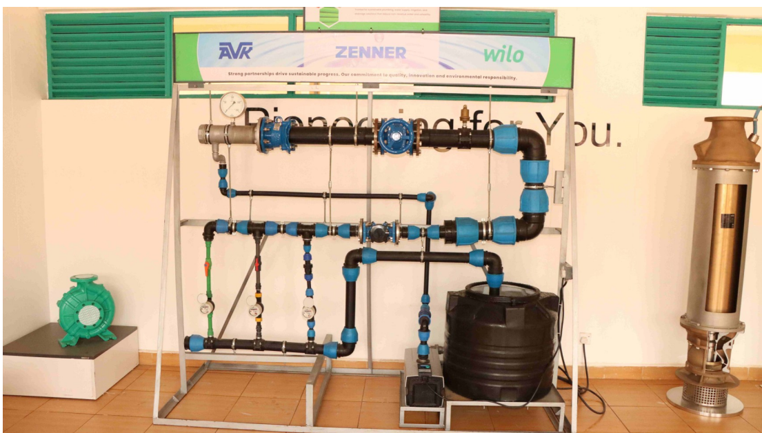
The newly installed Water Pressure Regulator/System at the Wilo Energy Efficiency Laboratory, a training platform on how proper pumps and pressure management can maintain water balance. Below- a member of the delegation inspects the system.
