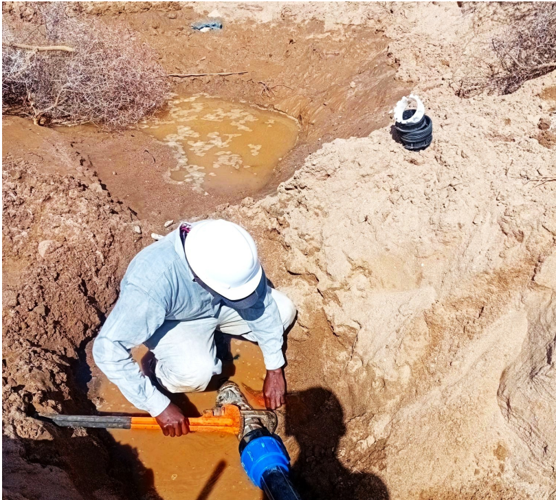
Bernard Mwaniki Mulwa fixing a water distribution pipe. He has been active in local plumbing and installation projects and is set to start his own water system installation and maintenance enterprise soon.
