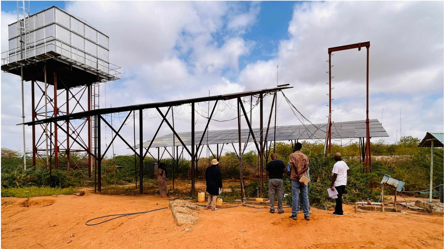
A solar-powered borehole in Daadab. Building local capacity in water supply operations, system maintenance, and solar technology management helps in strengthening of resilience for both refugee and host populations.
