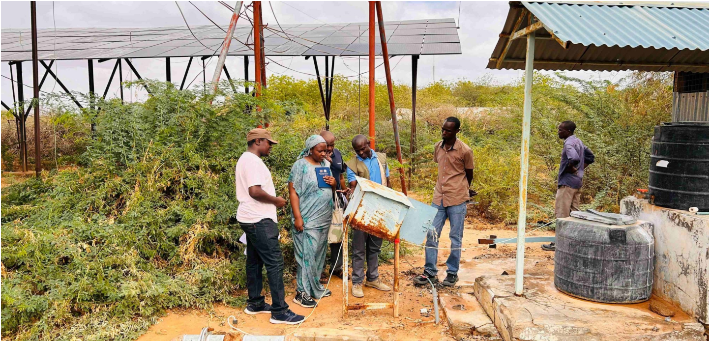
Training Needs Assessment (TNA) mission team inspects a solar-powered borehole in Korakora, Garissa County. There is the need for technical certification for local operators as a way of promoting long-term sustainability for the area water infrastructure.
