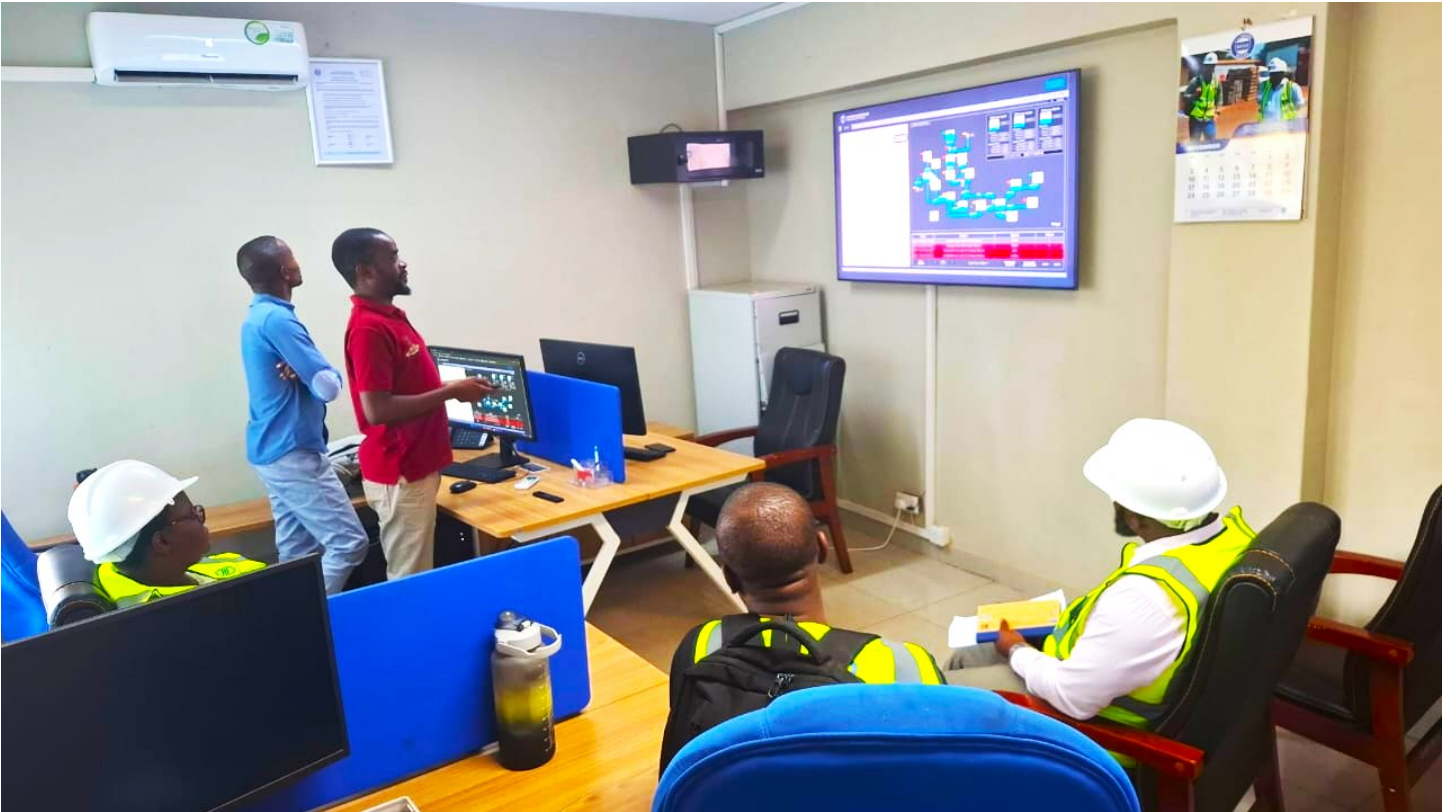
A Scada system at the Lilongwe Water Board call center, Malawi. According to a Follow-Up Report on Action Plan of the Malawi NRW Action Plan developed during the TCTP Phase I training, the utility has registered strong operational and capacity-building efficiency with the review indicating that 80% of actions in the plan are already completed.
