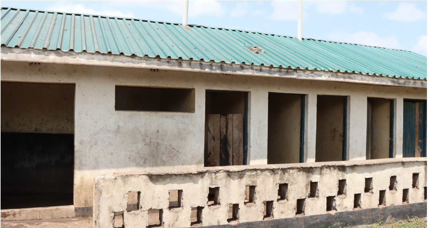
A block of pit latrines in a local school. Enhancing sanitation adoption requires attention not just to the physical availability of facilities but also to the underlying environmental conditions – especially water supply reliability – that influence household choices.
