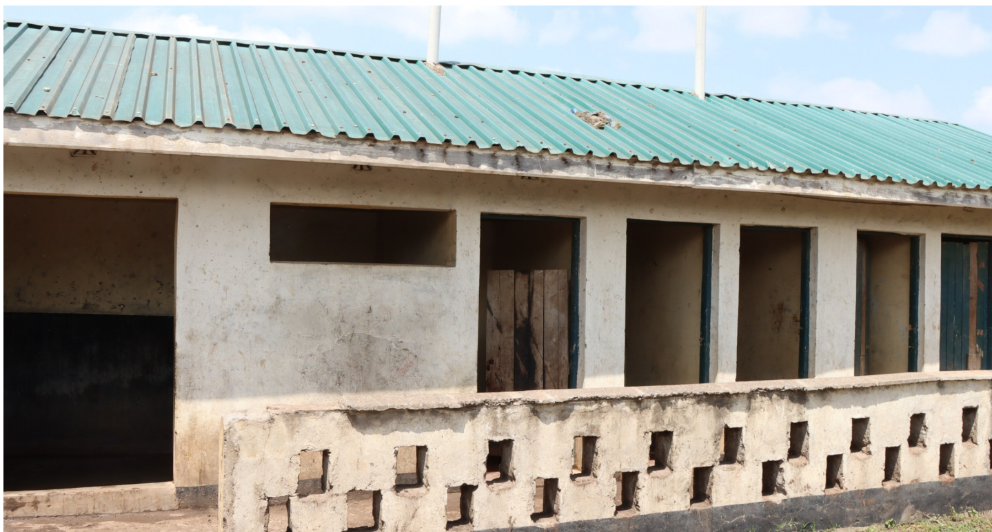
A block of pit latrines in a local school. Enhancing sanitation adoption requires attention not just to the physical availability of facilities but also to the underlying environmental conditions – especially water supply reliability – that influence household choices.
